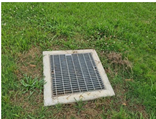
Stormwater drain in field
