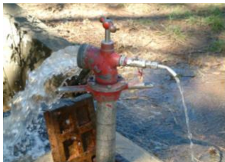
Figure 10 Standpipe with sampling tap
